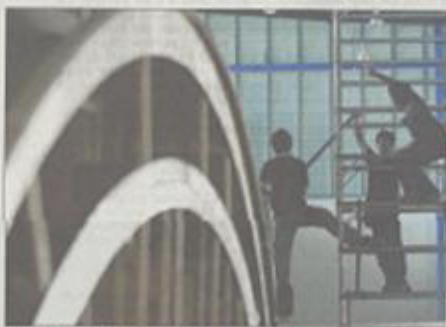
STEP BY STEP: Workers getting the exhibition hall ready: Teams are working seven days a week at the 30-ha site in Changi North.
